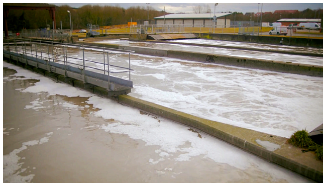
Northumbrian Water sewage works, Howden.
